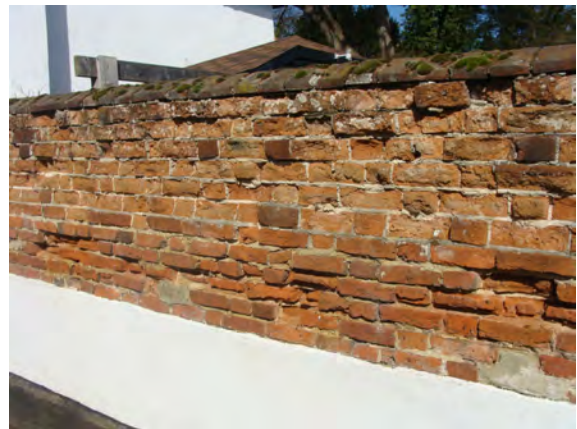
Picture 1.23 Red brick wall in need of restoration to Candle Cottage in strategic location on Stoney Lane
