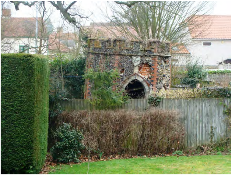
Picture 1.31 19th century folly in need of repair
