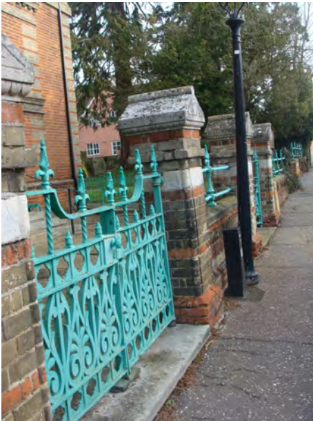
Picture 1.21 Fine 19th century railings to front of United Reformed Church in need of repair
