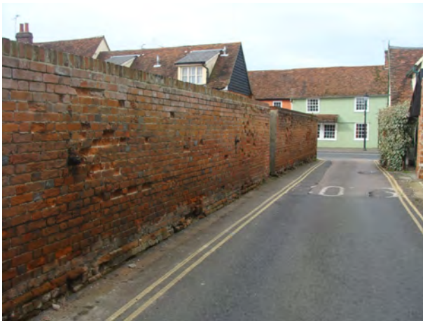
Picture 1.18 Boundary wall to Swan Hotel in need of repair
